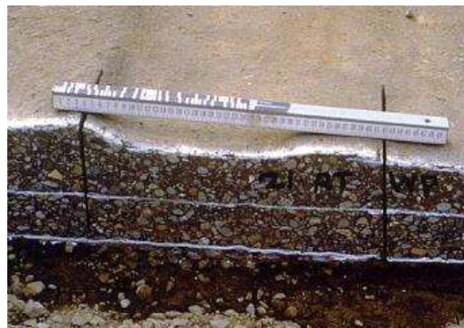
Figure 54. Example of rutting due to shear flow (Wes Track experiment)
