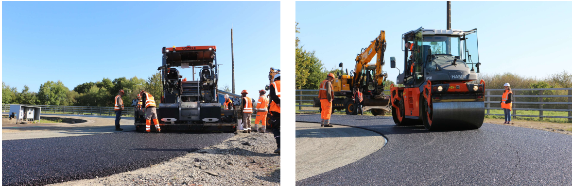
Figure 6. Pictures of paving operation for the 1 st layer of Peri-Urban section (BB 0/8)
