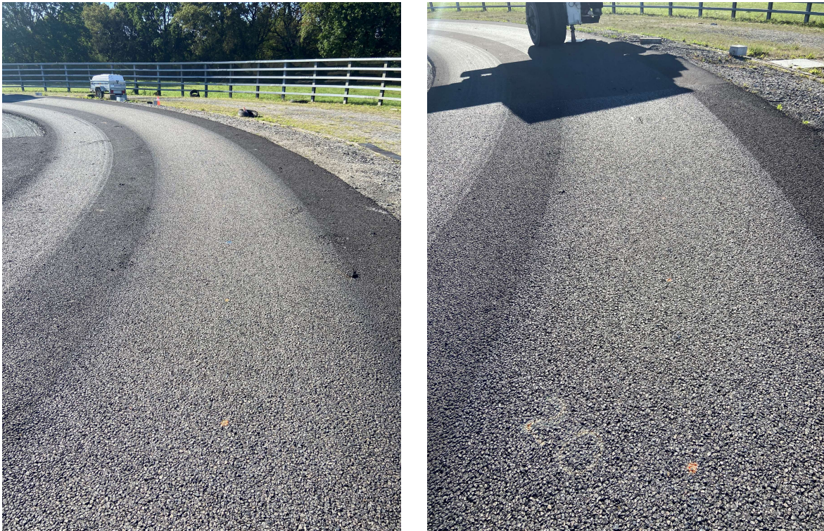
Figure 43. Photographs of the reference porous asphalt after 1 million load cycles
