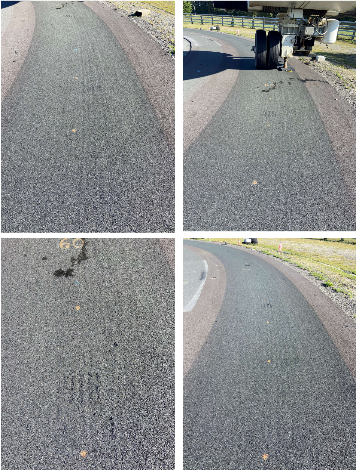
Figure 45. Photographs of the experimental urban mixture asphalt after 1 million load cycles
