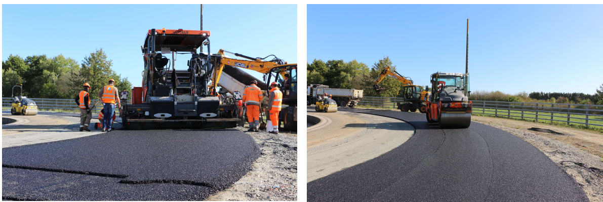
Figure 7. Pictures of paving operation for the 2 nd layer of Peri-Urban section (BB 0/4)
